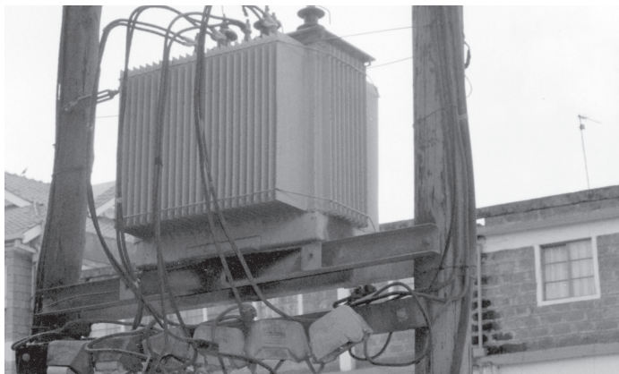
(c) A commercial step-down transformer
