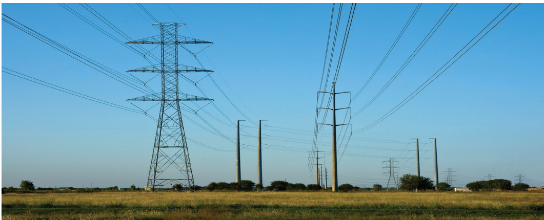
Fig. 8.1: Pylons and electricity transmission cables
